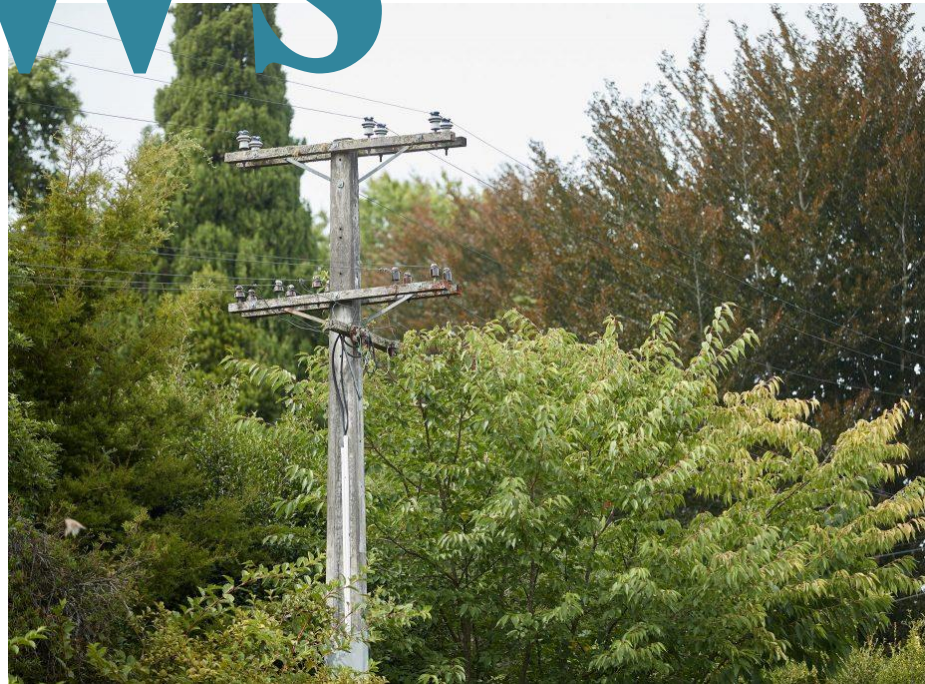
Example of vegetation too close to power lines
